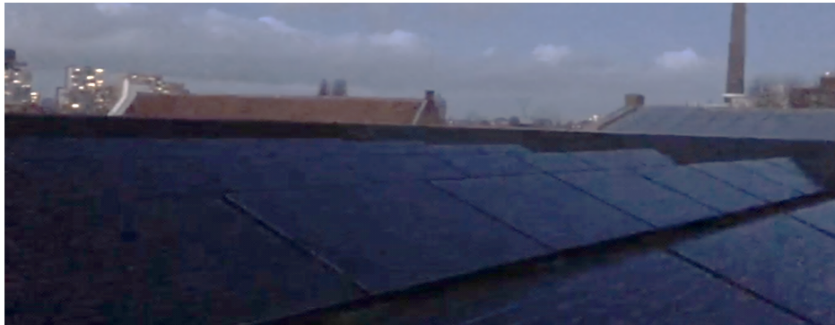
Picture 2: Solar panels on the roof of Gebr. De Nobel.
